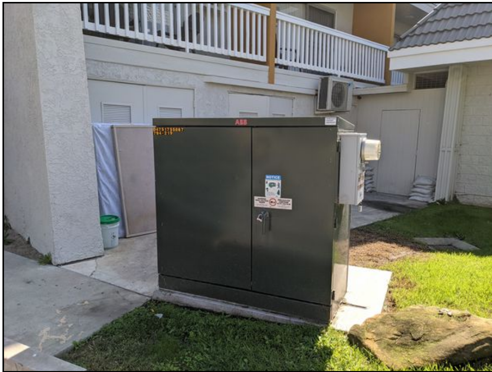
7 : Electrical transformer at hotel.
