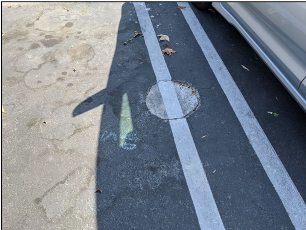
10 : Possible abandoned and plugged monitoring well in parking lot on south side of the site.
