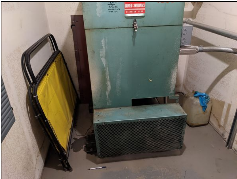
22 : Hydraulic elevator equipment within the hotel.
