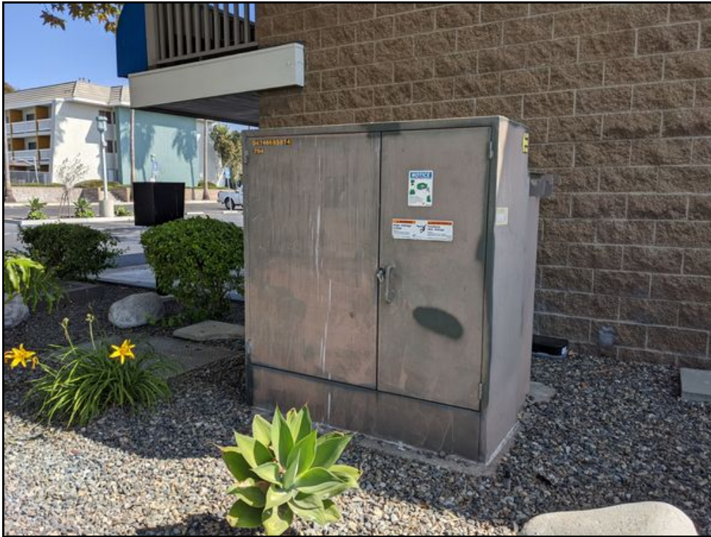
9 : Electrical transformer at 34553 Casitas Place.
