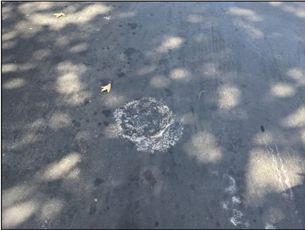
11 : Possible abandoned and plugged monitoring well in parking lot on south side of the site.
