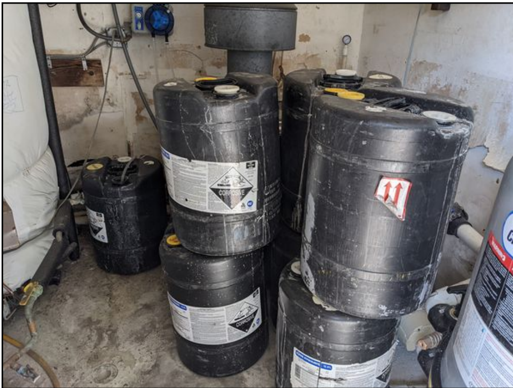
26 : Pool equipment and chemical storage room.
