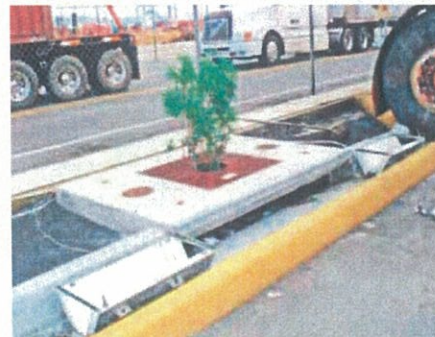
Filtterra® monitoring unit at an industrial port.
