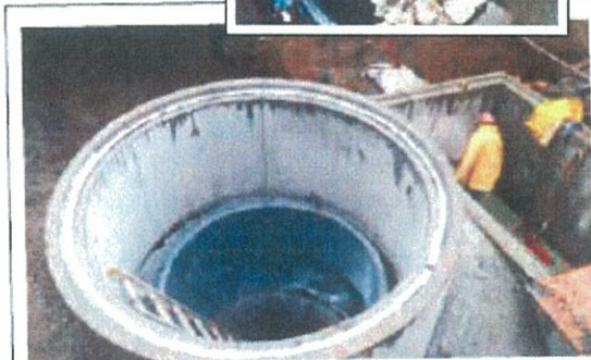
CDS unit installed to remove trash before entering Lake Meritt in Oakland, CA
