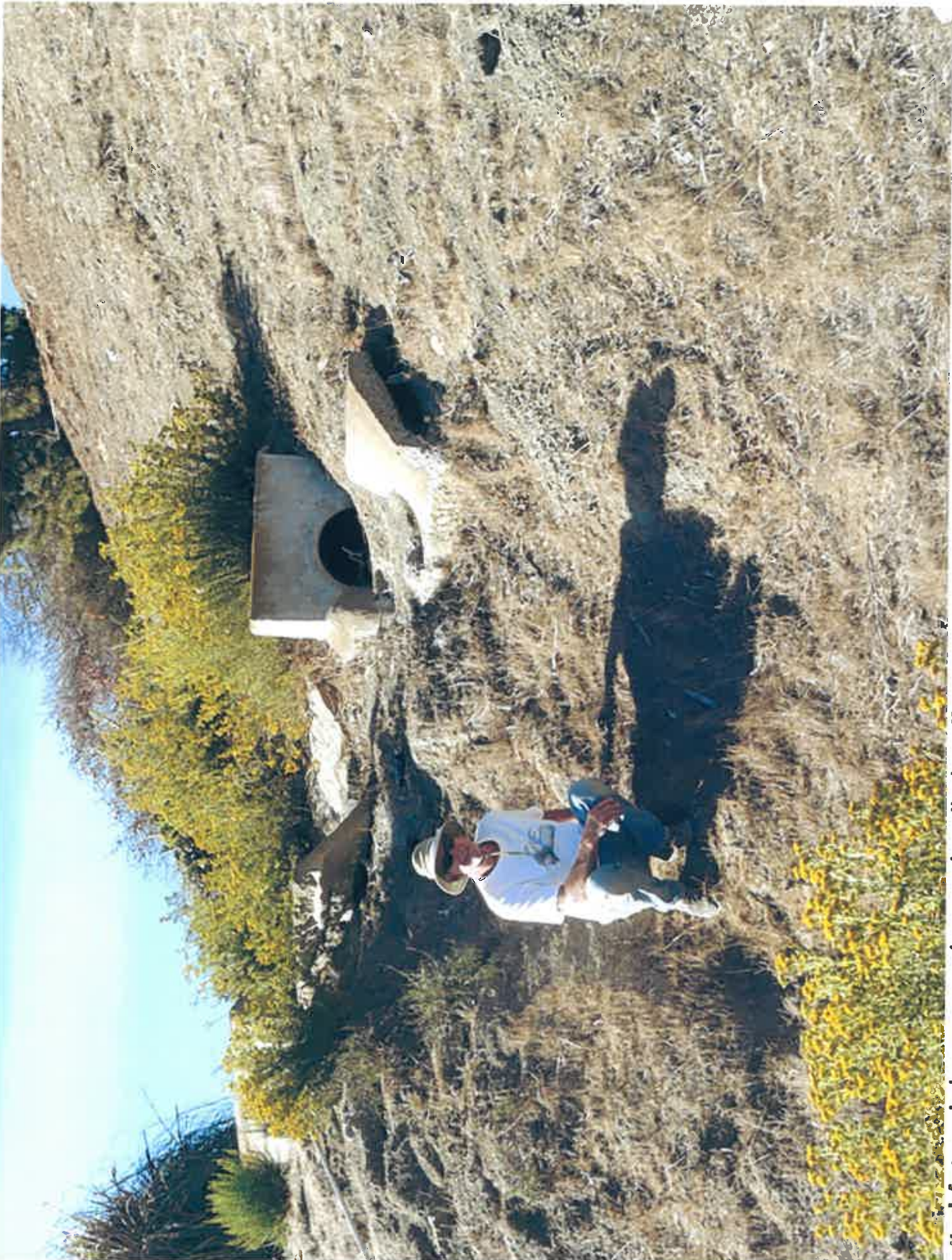
North-facing v-ditch system & outlet to nowhere (broken off, in disrepair): Pours off of the slope, does NOT connect/discharge into catch basin 250 below.
