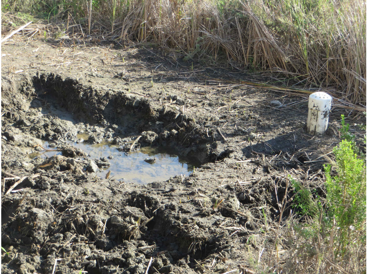
October 25, 2014. Standing water in percolation basin.
