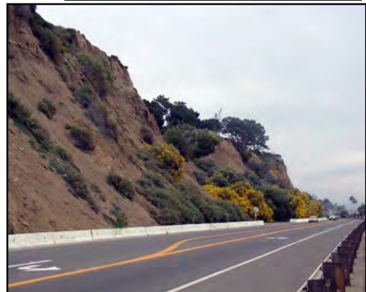
The instability of the Capistrano Bluffs is an ongoing concern. Regulations require that development be adequately set back from bluff edges, and traffic below must be protected
